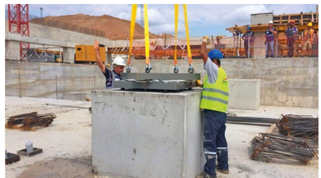
Figure 13 — Positioning of SIP D isolator on plinth in the cellar level below
